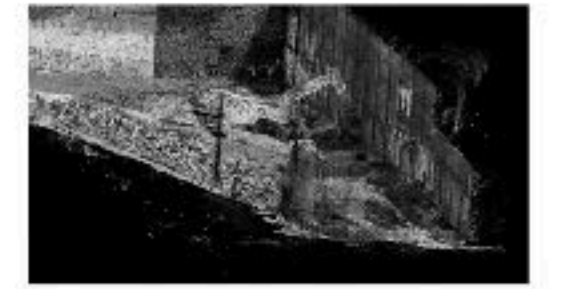
Figure 17.14 Point cloud segmentation: color clustering over point cloud geometries for rust detection.
